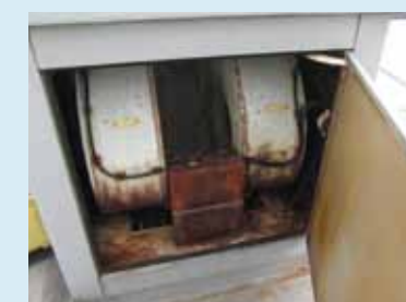
Failed and tired units
